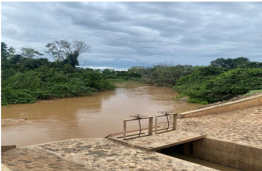
Fig. 7. Location of water intake at Wami River
