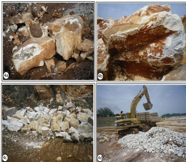
Fig. 4. Exploited materials, 4a and 4b: Blasted blocks in the order of 2 to 20 m, 4c: Treated blocks in the order of 20 to 35 cm, 4d: Crushed blocks
